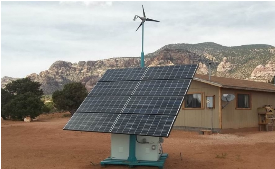
Residential Solar Hybrid Unit (photo from NTUA through energy.gov)
