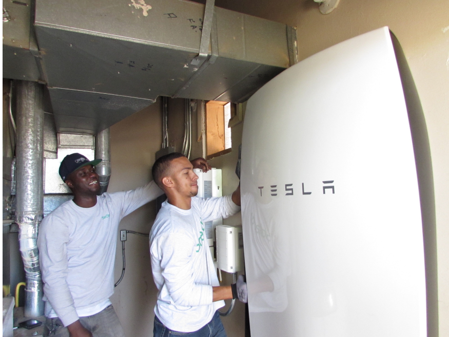
Solar City technicians installing the first Tesla Power Wall in Arizona at the Forest Lake Chapter House in July 2016 (photo by Stina Janssen)
